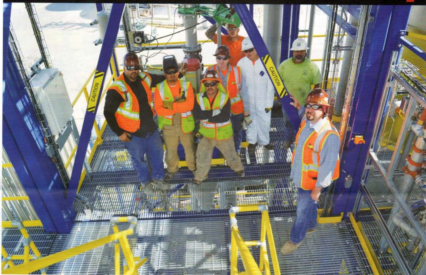
Part of the crew building the new chemical plant at the Port of Redwood City, from left Local 102 members Chris Boyce, Felipe Alvarez, Joel Escutia, Clifton Stewart, Kevin Roeh, Danny Bravo, Sixto Gutierrez (Laborers) and superintendent Joe Lawrence, also Local 102.
